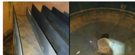
Stripper column internals
